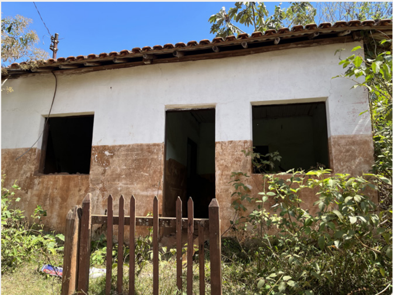
Mud line on a house hit by the Mariana tailings dam collapse, photo taken 27 August 2022
