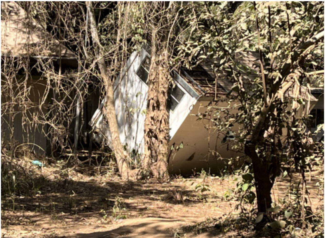
Building overturned by mud from the tailings dam collapse at Brumadinho, photo taken 18 August 2022
