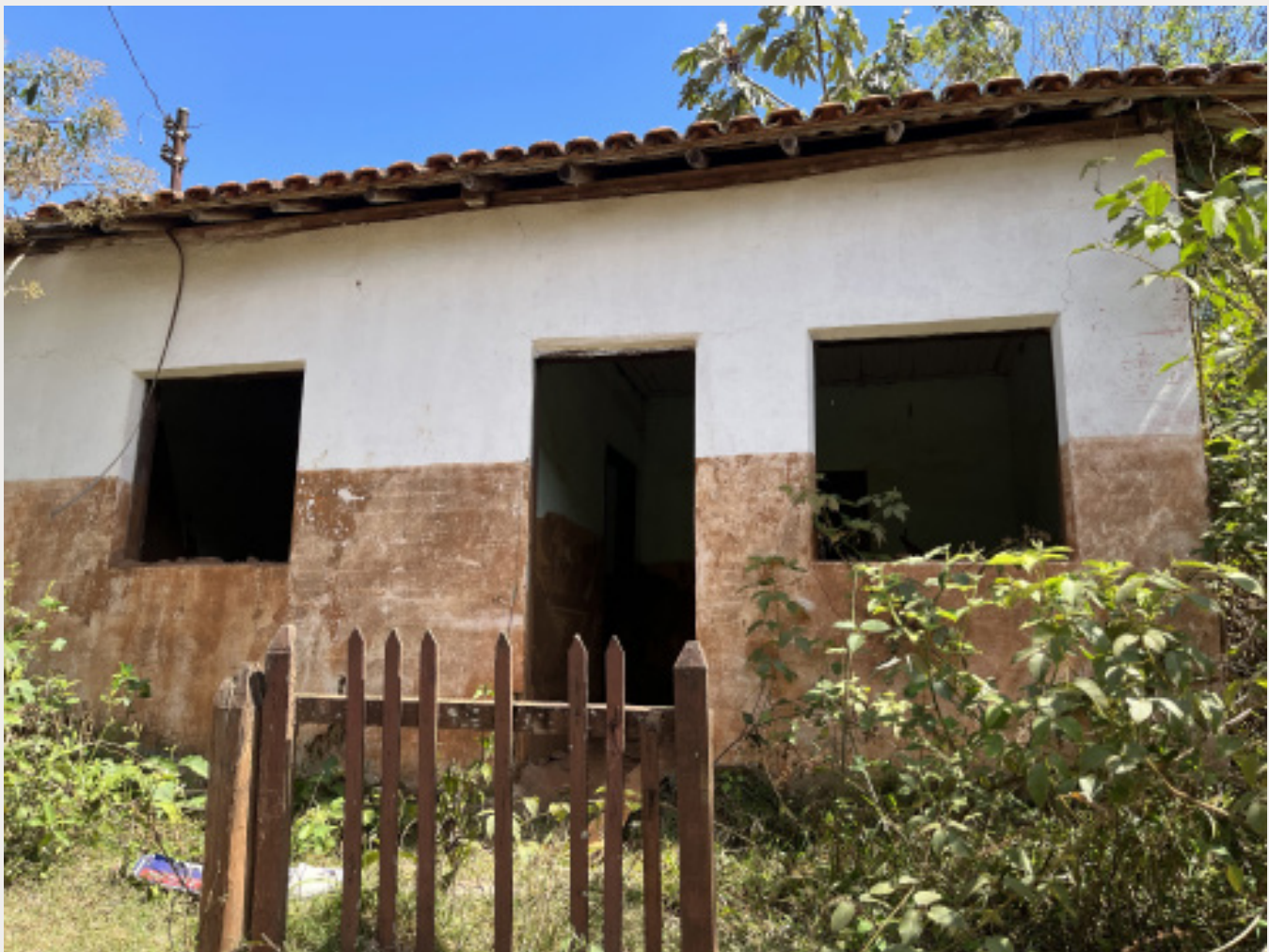
Mud line on a house hit by the Mariana tailings dam collapse, photo taken 27 August 2022
