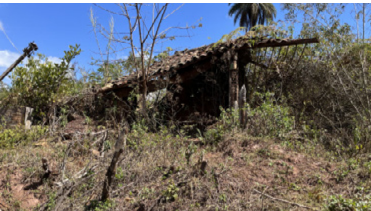
A house destroyed by mud in Mariana. As we descended the hill, the marks got higher and higher up the sides of the buildings until it was clear that the buildings had been covered by the mud, photo taken 27 August 2022
